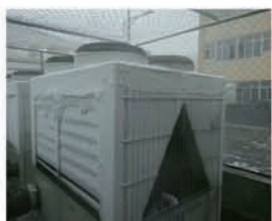
Heavy frost on electric air source heat pump
